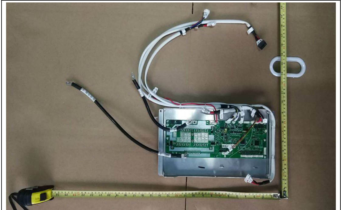
General view-2 of control panel
